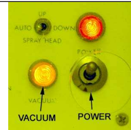
Fig. 1 Control Panel (DO NOT adjust any controls)
